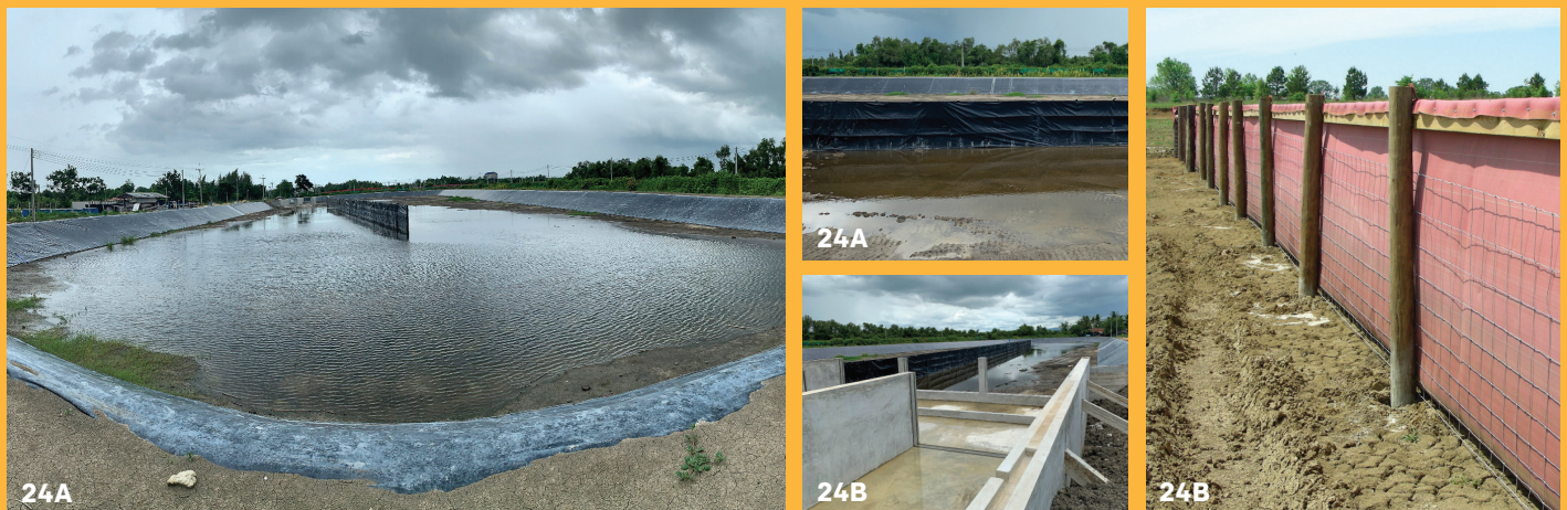
Figure 24A. Newly installed HDPE baffle walls 24B. Newly installed heavy nylon fabric baffle wall
