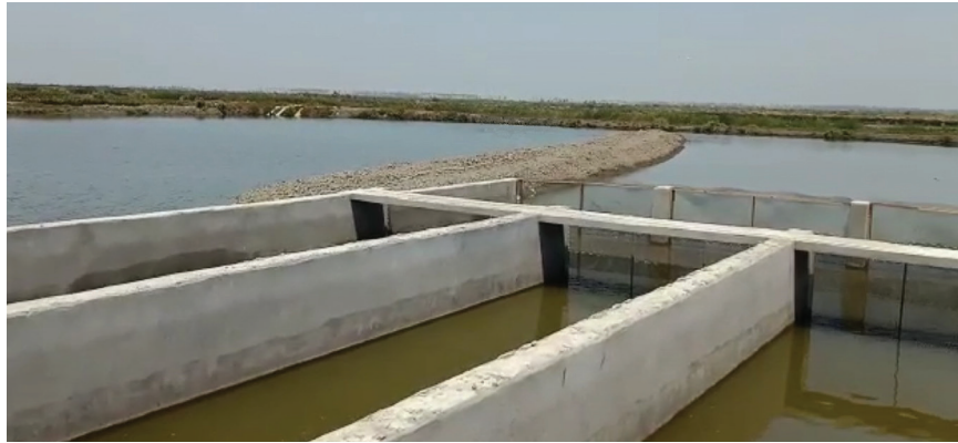
Figure 25. Earthen baffle levee (Mousa Wakileh)
