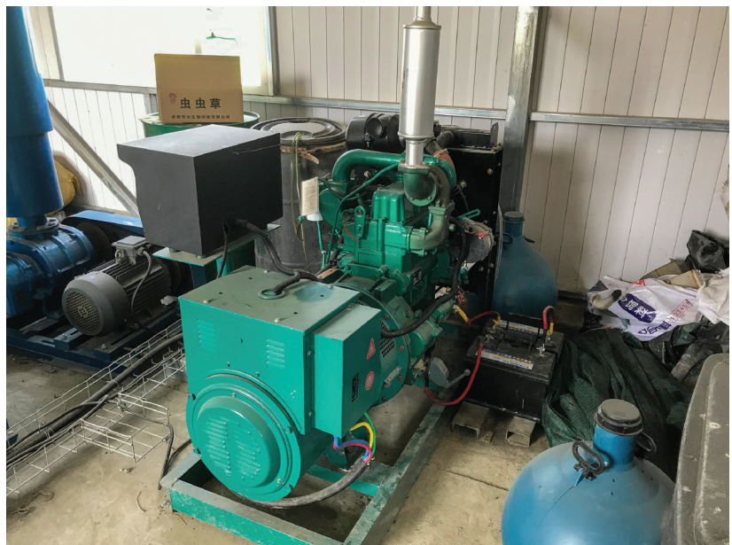
Figure 91. Auto-start generators should be inspected and tested weekly under operational load
