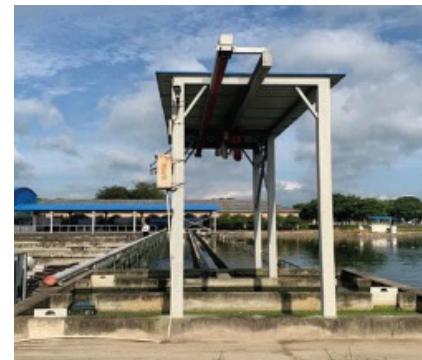
Figure 128. Early design of fish waste sedimentation tanks fixed in the pond; onshore designs are more efficient to operate
