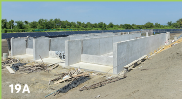
Figure 19A. Upper end knee wall at WWU attachment point 19B. Upper end knee wall at WWU attachment point 19C. QZ knee wall separating two solids removal zones
