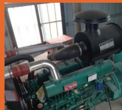
Figure 136. Auto-start backup electricity generator for IPRS operation
