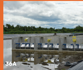
Figures 36A – C. Airlifts WhiteWater Units (WWUs) installed and operational
