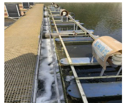
Figure 131. WhiteWater Units for IPRS operation
