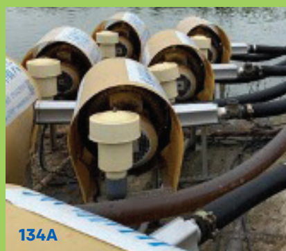
Figure 134A & B. Common blowers for IPRS operation in China
