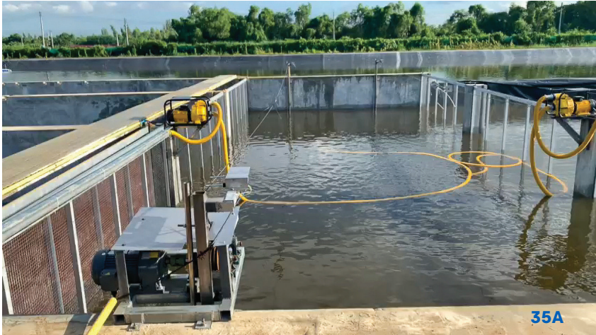
Figure 35A & B. Moving solids via hose and trough
