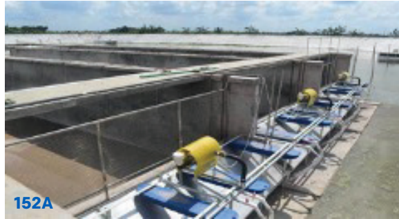
Figure 152A & B. Air lifts and bottom aeration system in place
