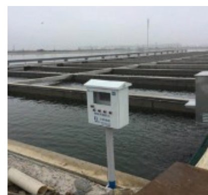
Figure 137. Auto monitoring and alarm system for IPRS operation
