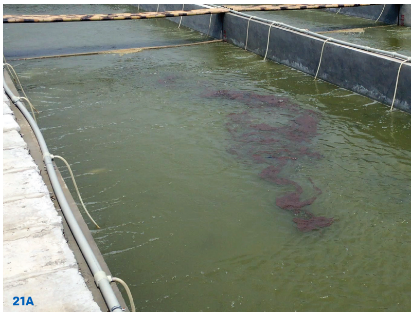
Figure 21A – C. Supplementary Aeration system in action
