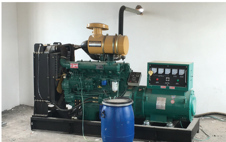
Figure 47A & B. Auto-start generators should be diesel, LNG, CNG or LP fueled
