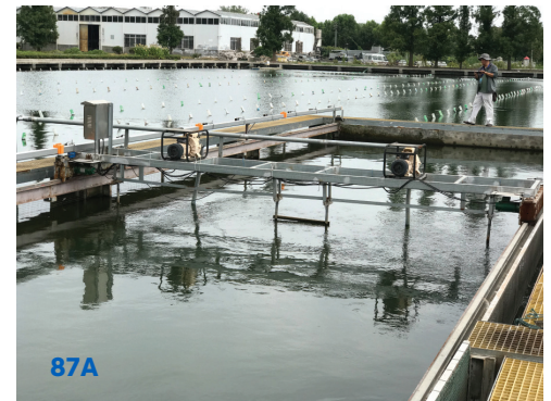
Figure 87A & B. Regular inspection of the solid waste removal system is critical
