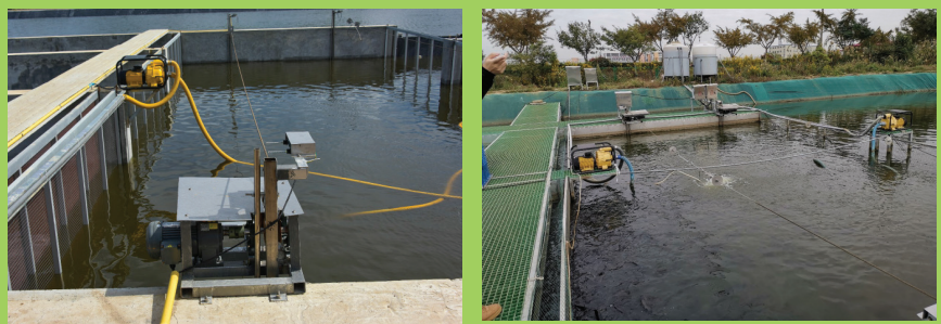
Figure 71. Cable operated solid waste removal system uses pumps to vacuum waste slurry to onshore storage tanks
