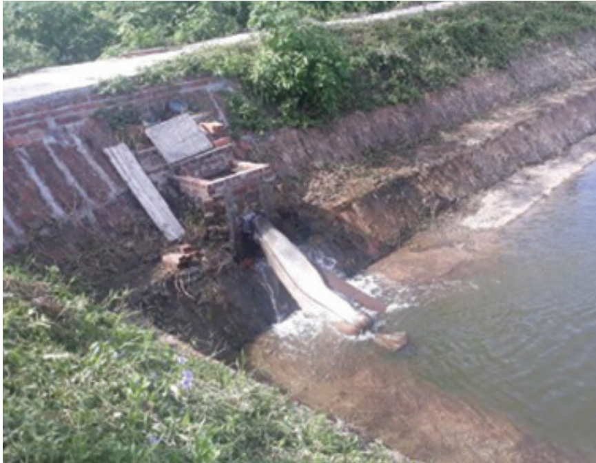
Figure 41. Saran sock filter for incoming water: Vietnam
